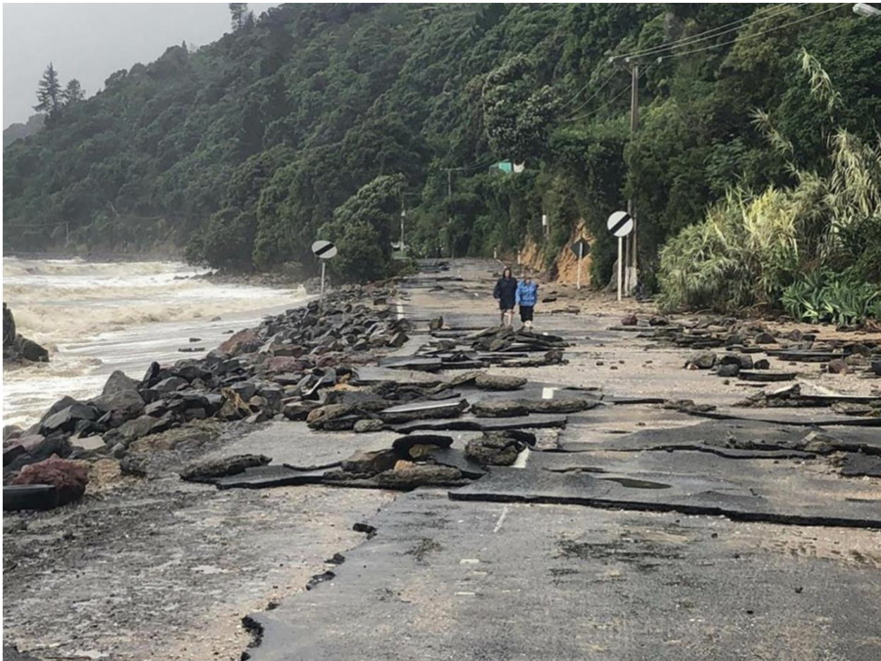
Figure 20 Storm damage on State Highway 25 along the Thames Coast from the January 2018 storm.
